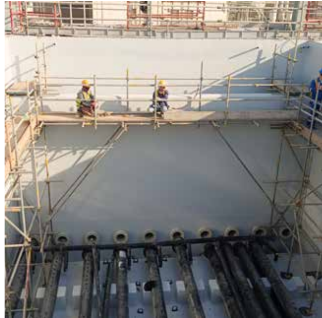
Desalinated potable water storage tank, Al Khobar, Saudi Arabia: 90,000 m 2 of Sikafloor®-161, Sikagard® PW.
