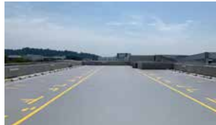
Exposed car park system
