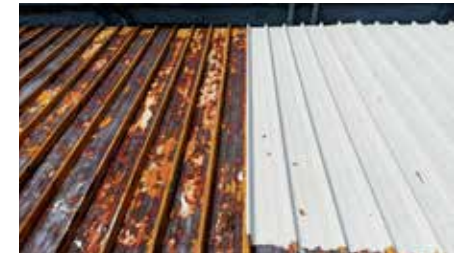
Corrosion steel roof
