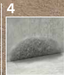
Leaking Areas of Voids i.e. Honeycombing
