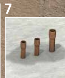
Leaking Penetrations i.e. Pipe Penetrations
