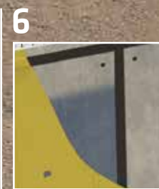
Leaking Compartment Membrane System
